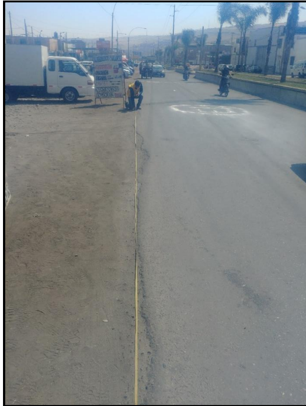
Desnivel carril berma
