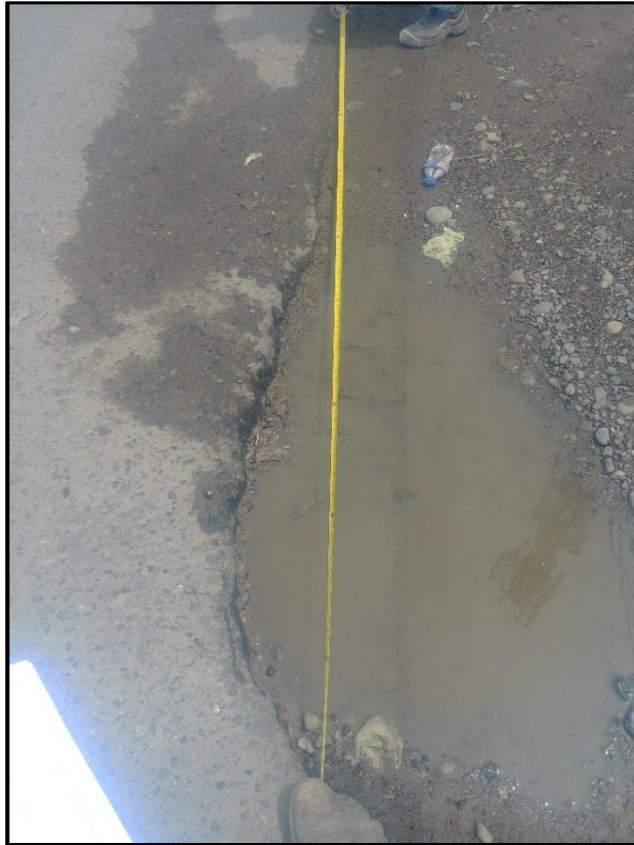
Desnivel carril berma
